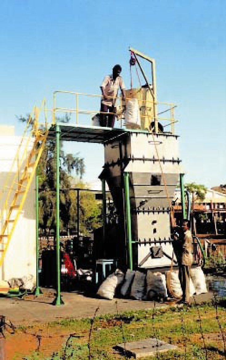
Biomass-gasifier power plant
